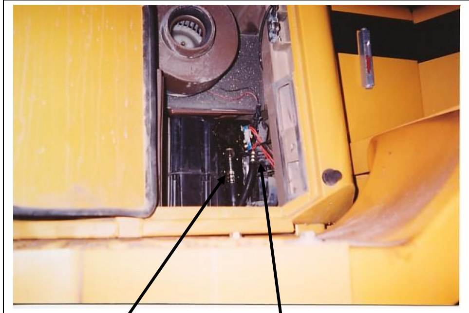
1/2" line connected to the evaporator outlet.
