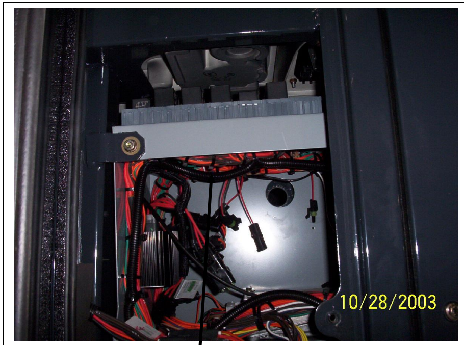
Clutch wire with loom re-installed running up the wire bundle towards the thermostat.
